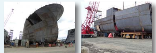
New Research Ships in construction (L) RV Neil Armstrong; (R) RV Sally Ride Photo Credits: WHOI & Scripps
